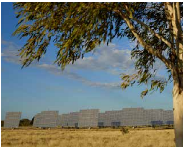
One of Alice Springs Airport's three solar facilities
