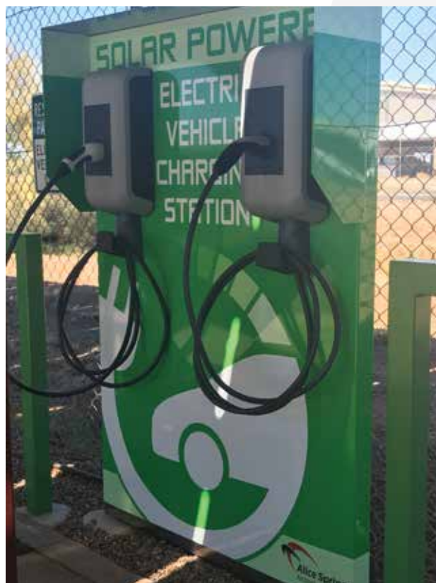
Solar powered vehicle recharge station at Alice Springs Airport
